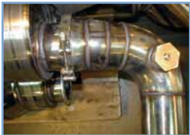
Figure 16 Smoke Port on Inlet Pipe
